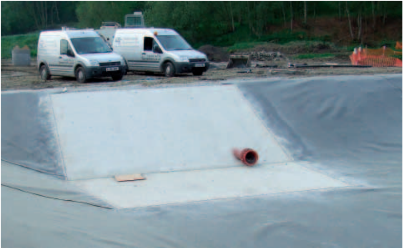
Drainage Lagoon Yorkshire
